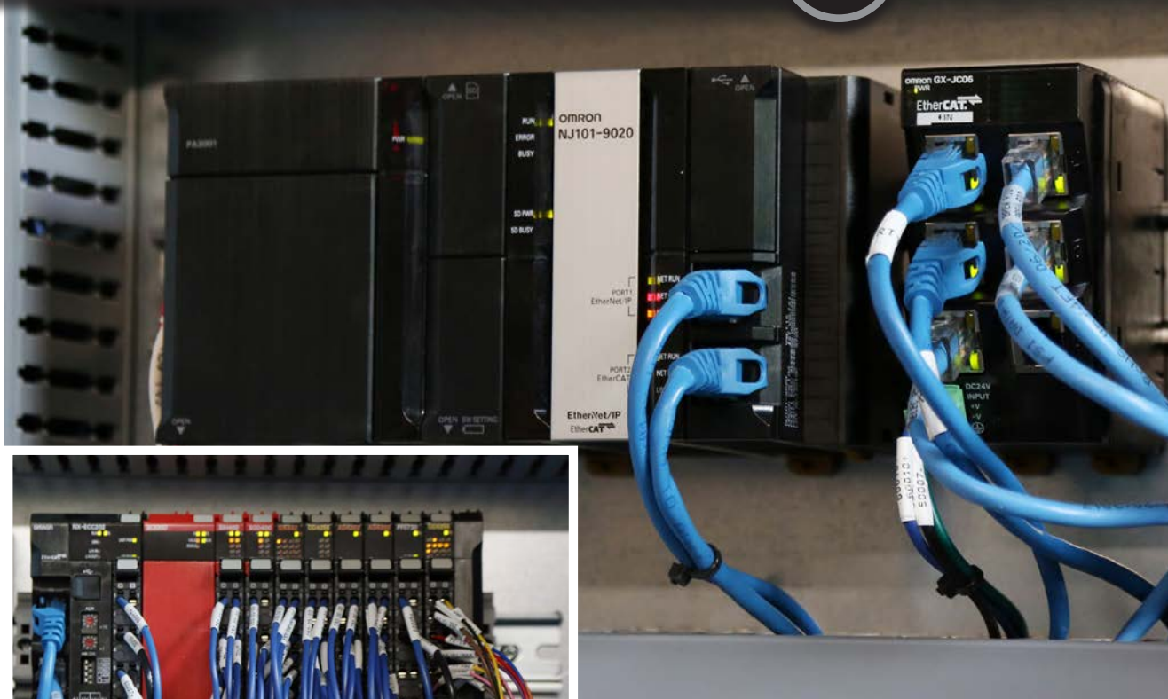
Omron controllers, I/O terminals and other automation devices were expertly configured and programmed by LSI Control Systems in a way that will enable the distillery to ramp up its production capacity and throughput down the road without any major downtime or interruptions.
