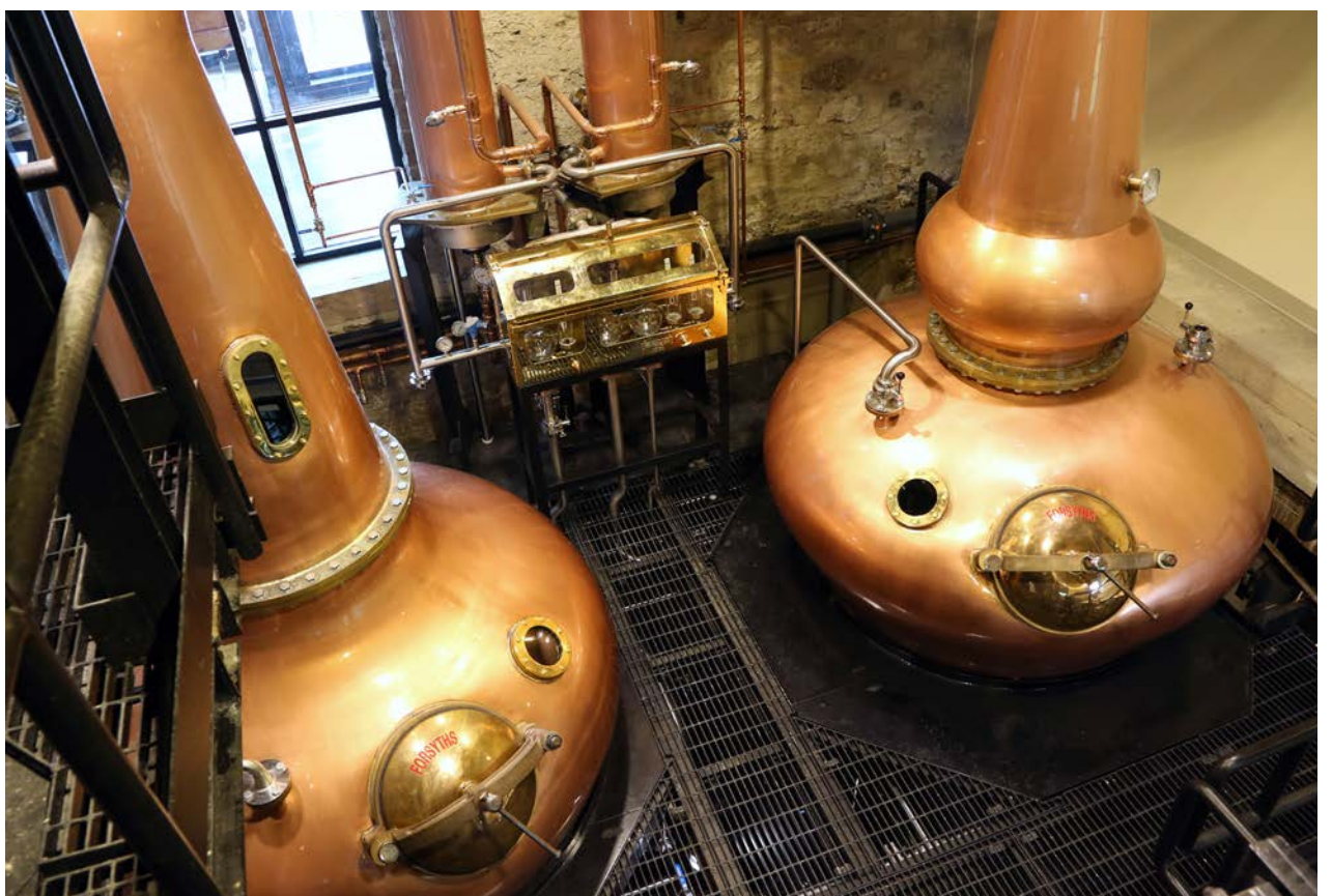
Measuring over three meters in height, the all-copper stills installed at the Spring Mill Distillery building were hand-crafted in Scotland by the world's leading and best-known distillation equipment manufacturer Forsyths, founded back in the 1890s.
